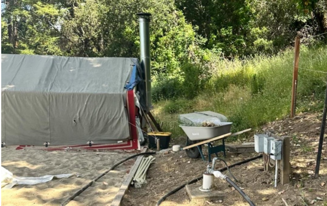
Figure 8a. Tent has chimney, presumably from wood stove. PVC electrical conduit is lying on the ground (unburied). All five photographs in Figure 8a-8e were from Hipcamp advertisements of campgrounds in Santa Cruz County.
