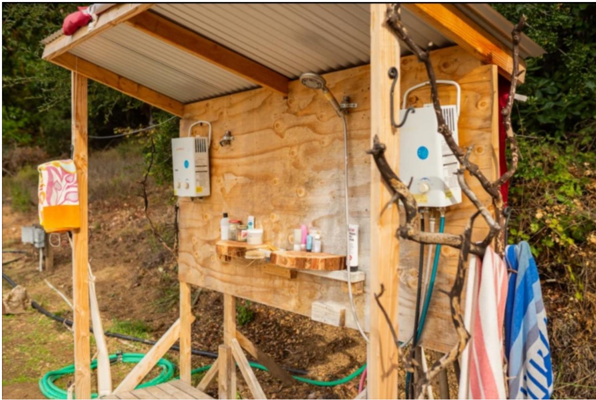
Figure 8b. Outdoor shower with propane heaters and electrical conduit on the ground. The propane heater at the right is suspended loosely by a single nail.
